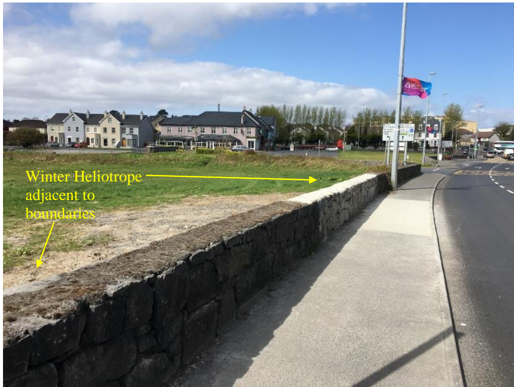
Photo 12.6: Showing the approach to Moneenageisha junction on the Dublin Road. Note the disturbed ground and wall repairs.
